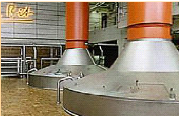
Brewing Is A Classic Hybrid Industry Combining Elements Of Process and Discrete Applications
