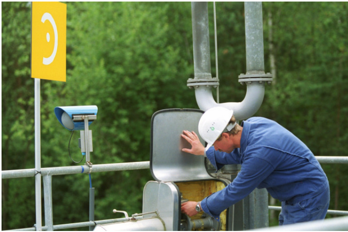
PROFIBUS Allows CenterPoint to Centralize Data Collection for Better Prediction and Elimination of Premature Valve Failures
